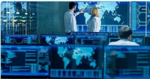
Enterprise Data Center
