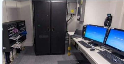
School Server Room
