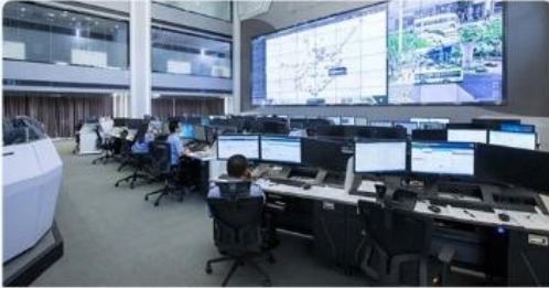
Surveillance Control Room
